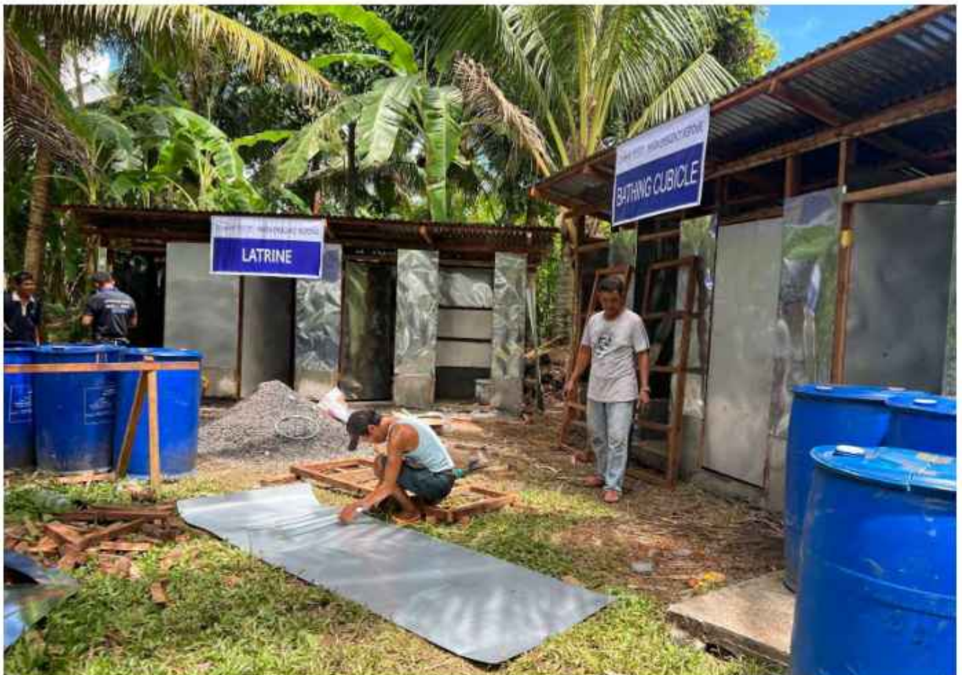
Construction of latrines and bathing cubicles in the Philippines in a cash-for-work programme as part of the response to the Mayon volcanic eruption. © IOM 2023/Christine ARMENTA
