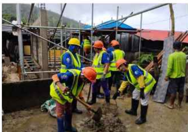
Participants in CFW as part of the typhoon resilient shelter project in the Philippines. © IOM 2023/Lorna HILARIO
